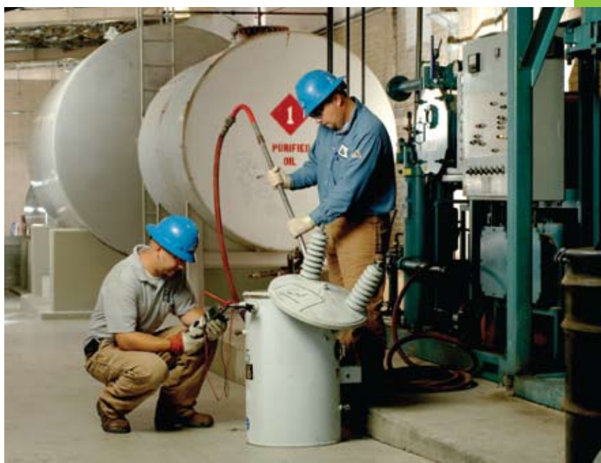
NES employees (left to right) William Friedberg and Larry Chunn recycle the oil found in a transformer. In most cases, the oil recycled on-site is cleaner than the original oil.
