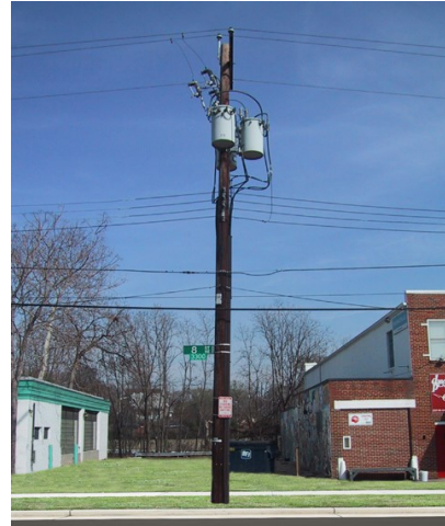
Figure 1B: Utility pole (Overhead System)
