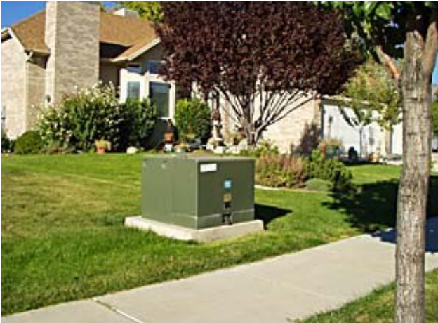
Figure 1A: Pad-mounted Equipment (Underground System)
